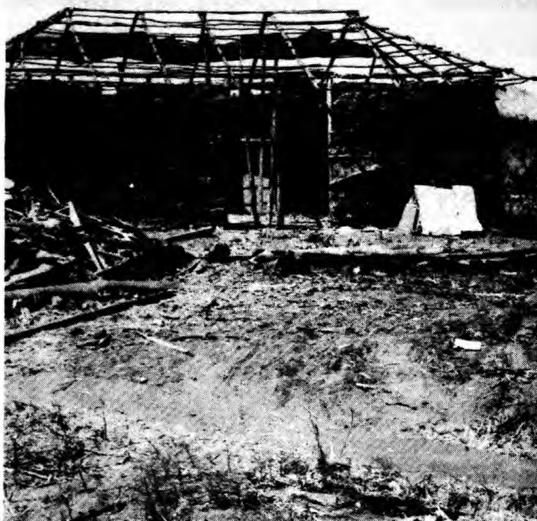
Church building going up at Kamai. The members are doing the work themselves. The plot of ground was given by one of the chief men of the village.
